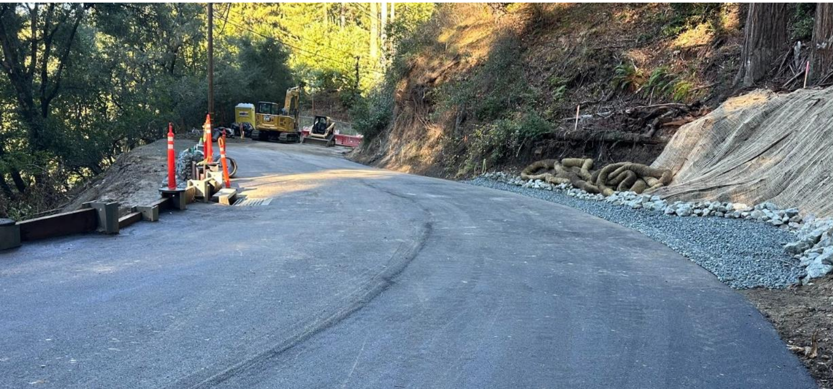
Figure 2-11: Bean Creek Road Erosion Control
